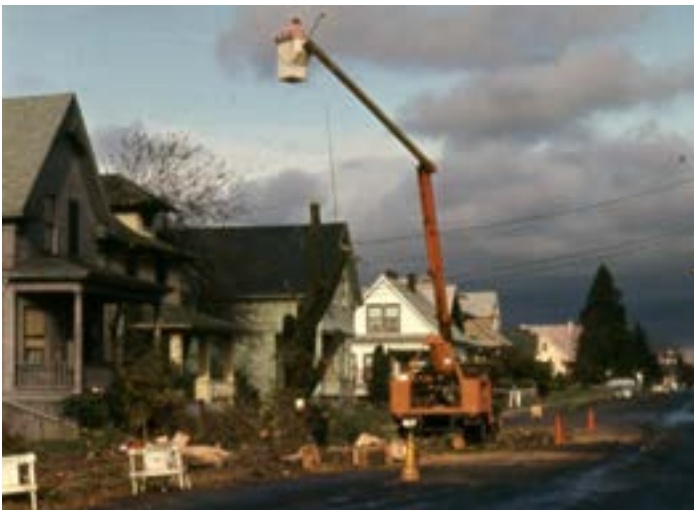
After delays from the Columbus Day Storm, Portland General Electric and Pacific Power and Light crews conducted major tree removals prior to the replanting in the project area during the spring of 1963. City of Portland Archives, A2010-003.
